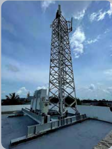
Gambar 13. Glass Fiber Reinforced Polymer Tower
